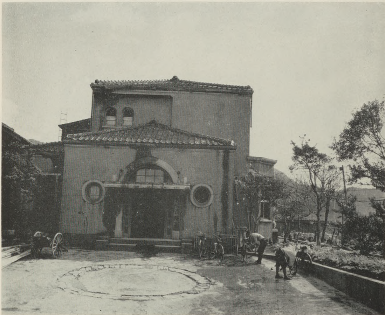
Photo 9. Nagasaki fire department headquarters building. No space provided to house fire equipment. Partially damaged by atomic bomb, 9 August 1945.
